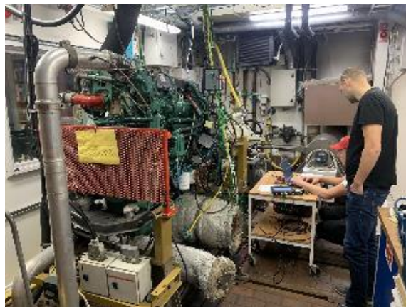
4 | Development and testing of the methanol injection control system
